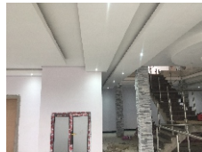
Electrical and Electronic Services Installations Fire alarm system 5kva Solar System
