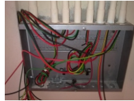
Electrical Services Installations
